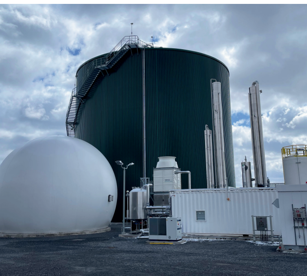
Dairy manure anaerobic digester to biomethane system installed in 2023.
